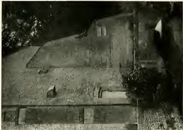
OLD CRIST MILL AT BIBURY The large buttress is supported by a stone arch which spans to mill race
